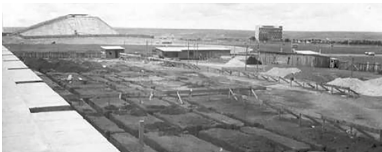
Start of construction on headquarters for Touring Club in Brasília, 1964. Source: Touring Club do Brasil Collection
