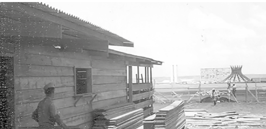
Construction shed at Touring Club headquarters, Brasília, 1964. Source: Touring Club do Brasil Collection
