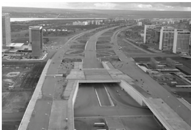
Start of construction, with connecting walkway already completed, 1965. Source: Public Archive of Federal District
